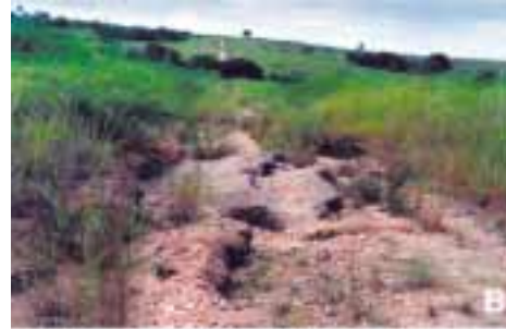
Picture 'B' (20) shows a surfaced road that has become so damaged that it cannot be traversed in an ordinary vehicle.
