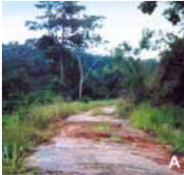
Picture 'A' shows a broken road surface. Mines are often concealed in the potholes. They may also be concealed under the thin tar by melting areas and putting the soft tar back on top of mines.
